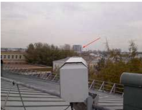
FSO equipment M1 ARTOLINK (MOSTCOM) in Moscow - distance 0.8 km
